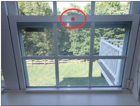
Window - Stuck Closed
