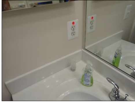
Cracked Outlet - Bathroom
