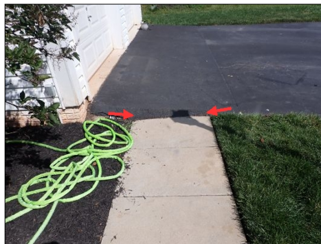
Walkway - Trip Hazard
