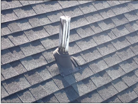
Radon Exhaust Pipe
