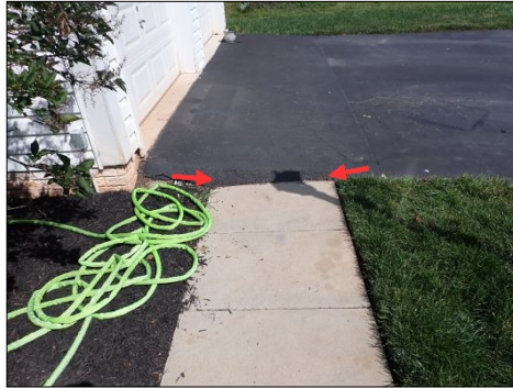
Walkway - Trip Hazard
