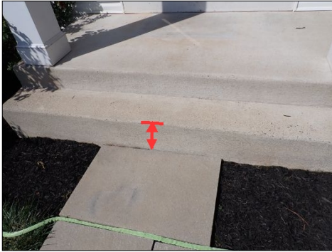
Concrete Steps - Trip Hazard
