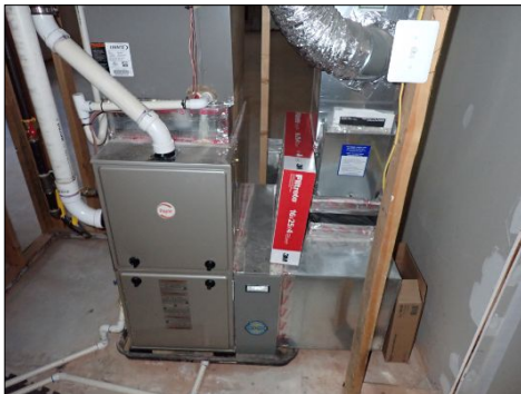
Gas Furnace - Unit #1
