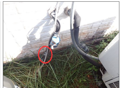
HVAC Refrigerant Lines
