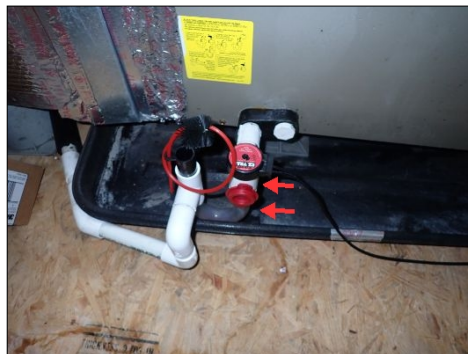
Condensation Drain Maintenance
