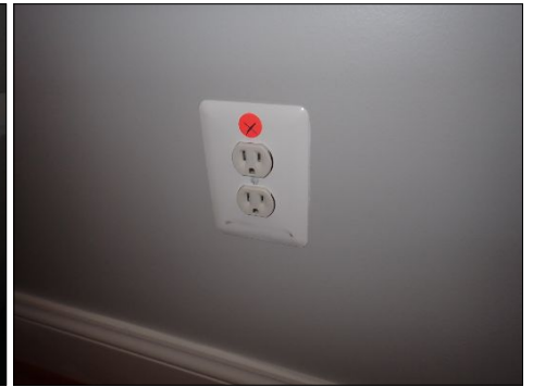
Cracked Outlet - Dining
