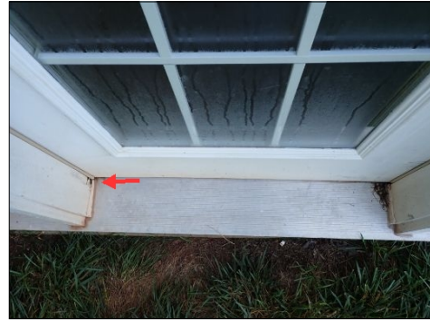
Rotted / Damaged Trim
