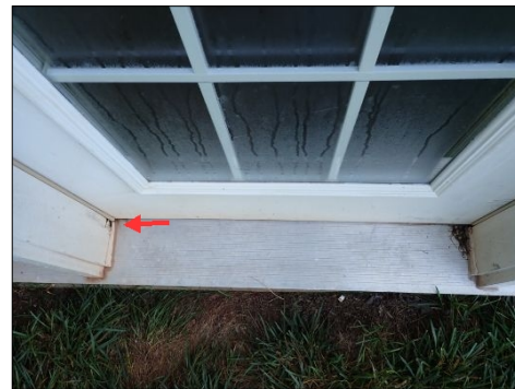
Rotted / Damaged Trim
