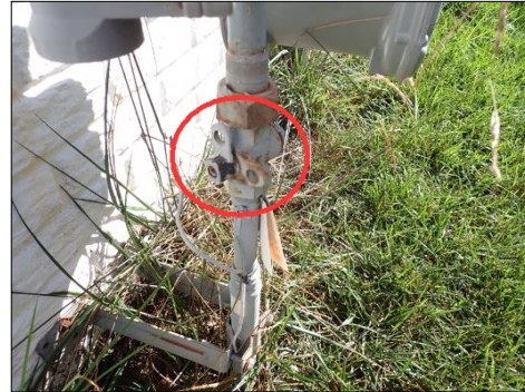
Main Gas Valve
