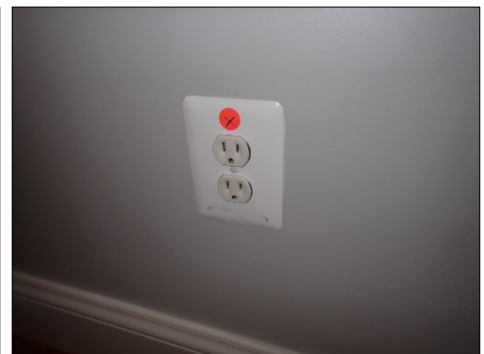
Cracked Outlet - Dining
