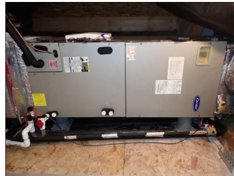
Heat Pump - Air Handler - Unit #2
