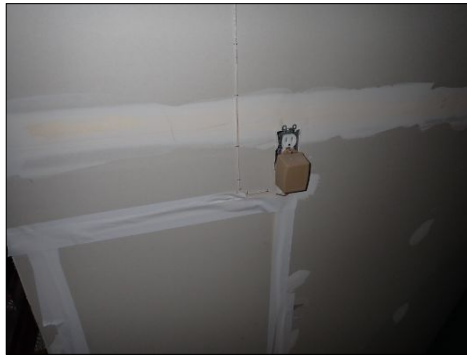
Open Electrical - Basement
