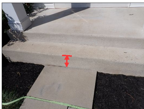
Concrete Steps - Trip Hazard
