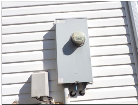
Underground Service to Meter
