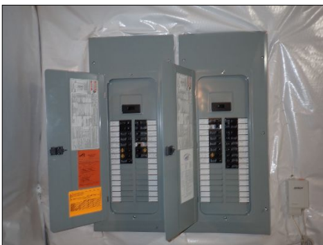
Main Electrical Panels
