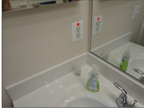
Cracked Outlet - Bathroom
