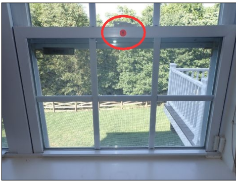
Window - Stuck Closed
