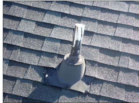
Plumbing Vent Pipe
