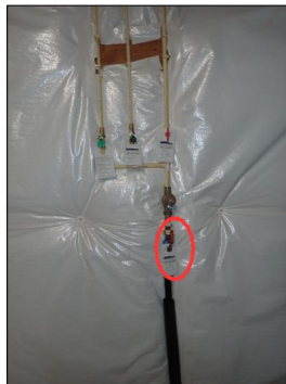
Main Water Valve
