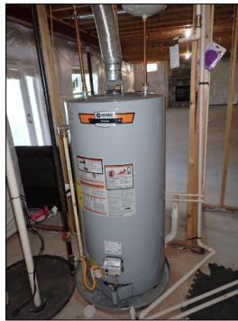
Gas Water Heater
