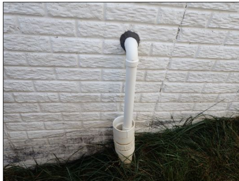
Sump Pump Discharge
