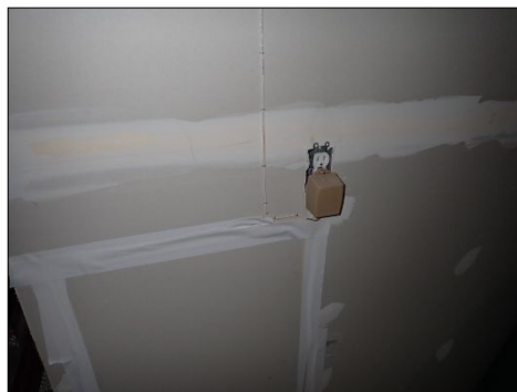
Open Electrical - Basement
